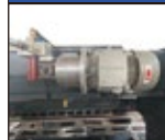
Germany SIEMENS Main Motor
